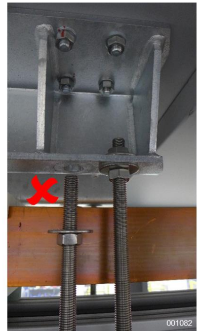
Loose screw connection
